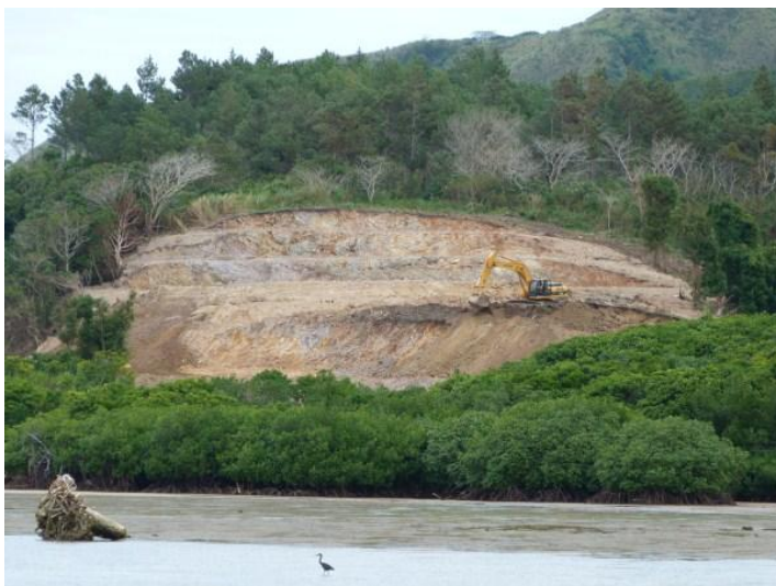
A JCB, just visible against the bare, newly-excavated earth, is one of two diggers being used to lower a coastal mountain to create a flat, tiered site for the resettlement of Narikoso village
