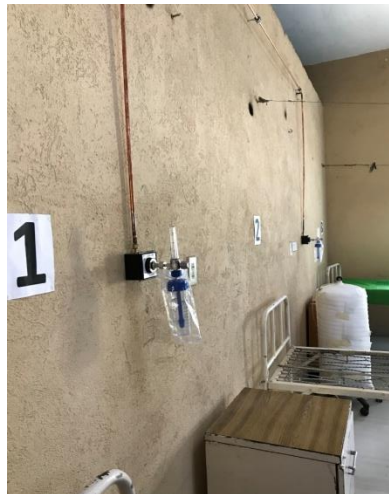
Oxygen Outlets in the Ward
