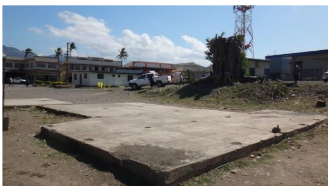
Rakiraki Market, Fiji: Foundations of the vendors' accommodation centre and the stub of the tree (silhouetted) that collapsed on the building are all that remained after the destruction of Cyclone Winston.
